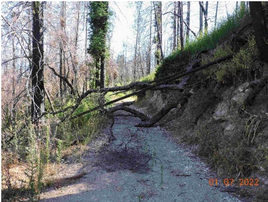
Photo 112. Bypass road = mile 2.75. The only downed tree obstructing road on 1 July.
