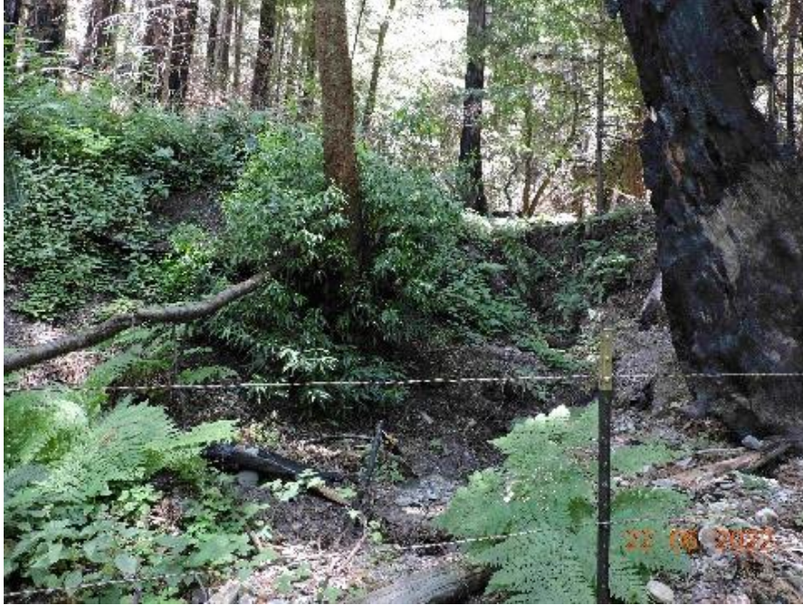
Photo 15. Mile 2.15. Eroded seasonal channel upslope of road.
