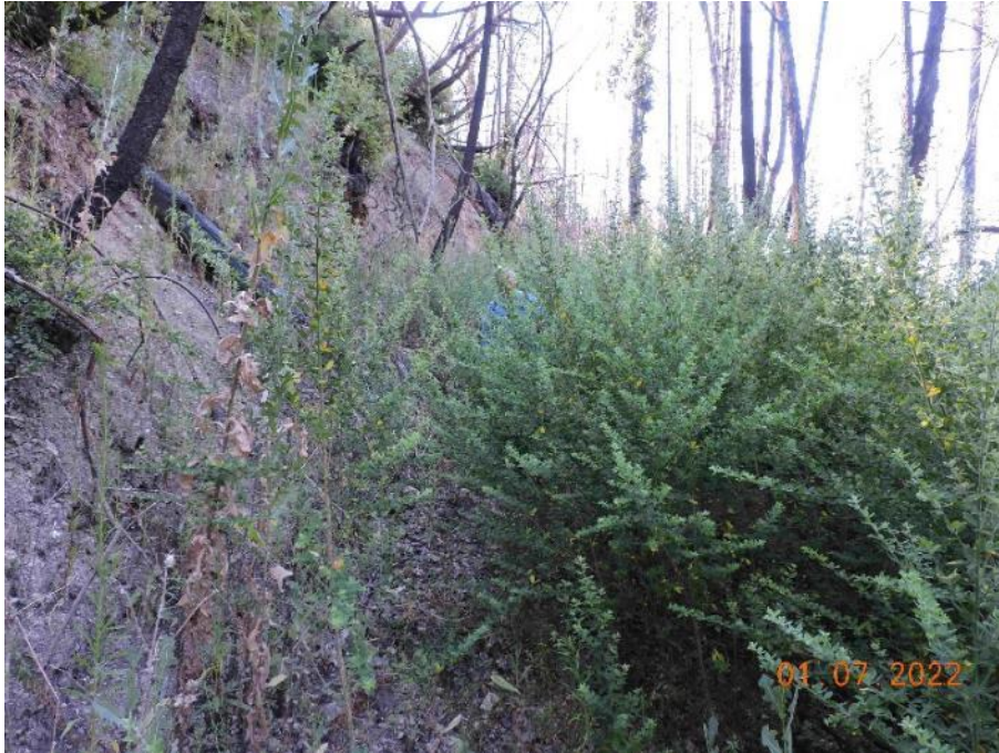
Photo 125. Bypass road, mile=2.9. Tall and dense blue blossom ceanothus and French broom in road. High cut bank shows no evidence of erosion.
