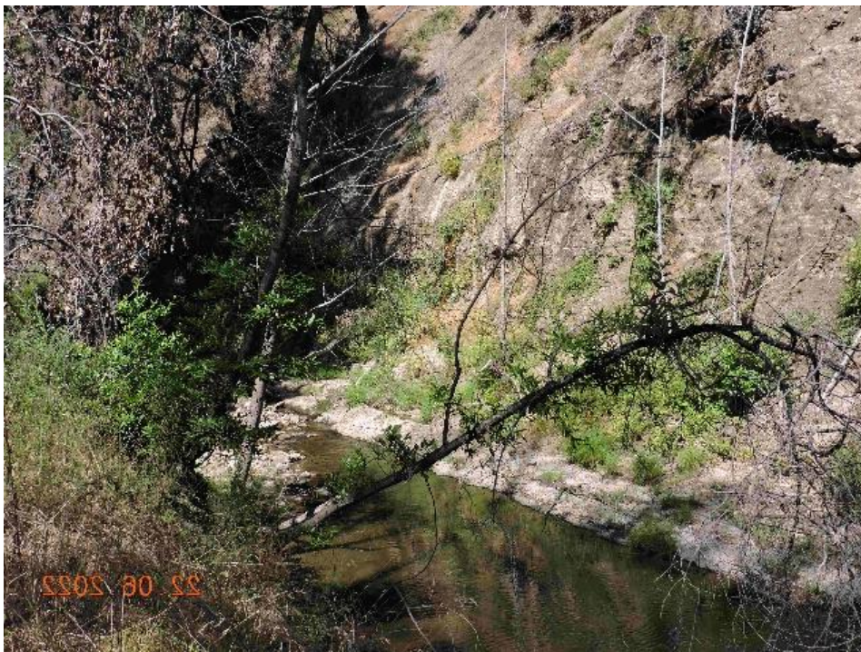
Photo 52. Mile 3.05+, Camp Herbert. Steep eroded slope and substantially filled pool from lower west slope erosion.
