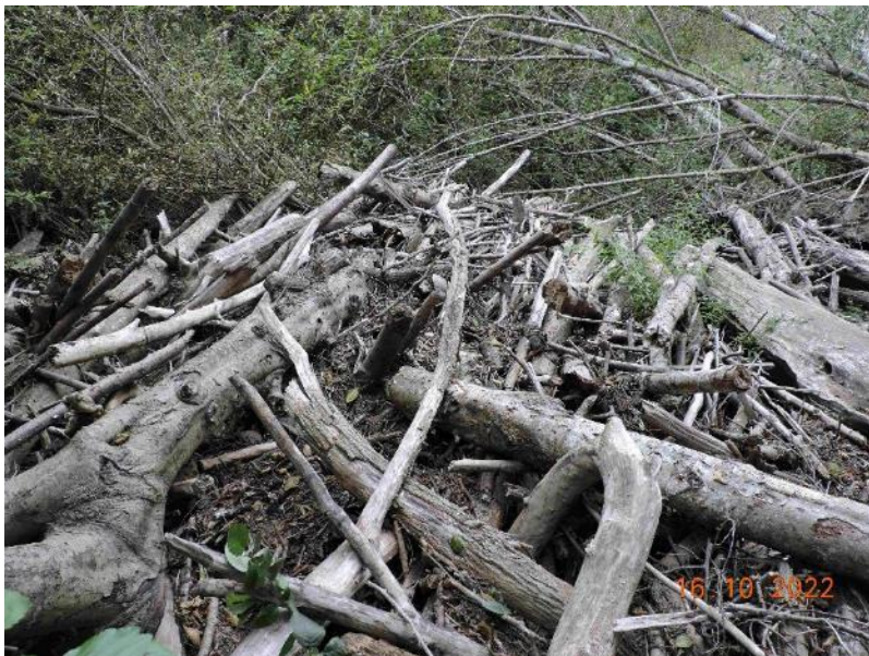
Photo 2. The logjam at mile 0.65 also extends 45 ft across the left bank flood plain, so even most high flows aren't likely to bypass the jam.
